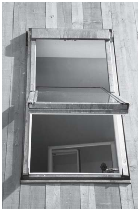
Fig. 302: Close-up of window The ventilation flap and roller blind are behind the fascia panel at the top.
