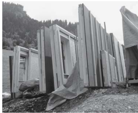
Fig. 45: Platform frame elements prior to erection Bearth & Deplazes: private house (Willimann), Sevegin (CH), 1998
