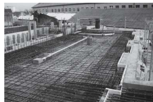
Fig. 52: 1st floor slab The returns in the slab edge elements indicate the positions of the French windows.
