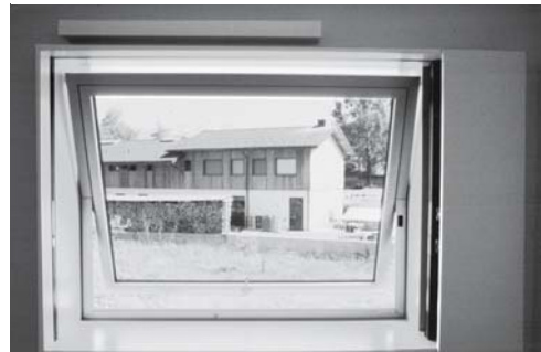
Fig. 122: Horizontal pivot window from inside
