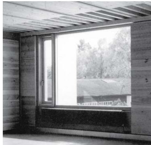
Fig. 280: Window The window is fitted directly into the structural frame. A narrow opening light for ventilation has been included instead of just providing a large undivided glazed area.
