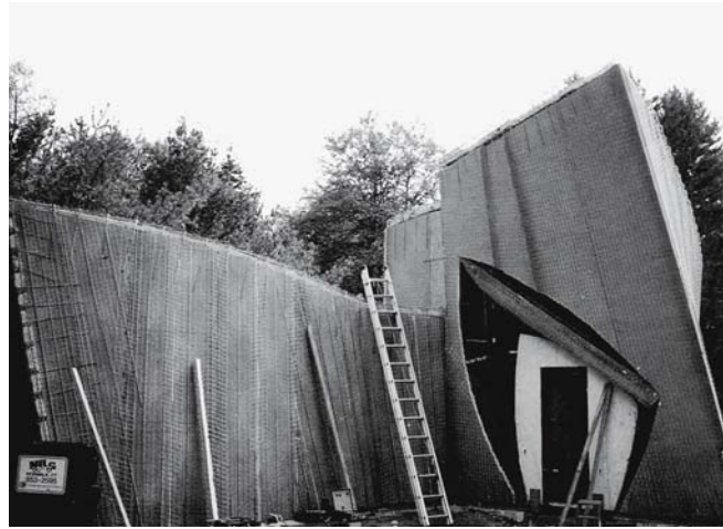
4 Cut-out for large entrance opening (note the difference between this and photo 3). Edges reinforced with additional bars.
