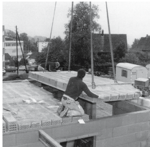
Fig. 1: Top: hollow clay blocks and reinforced concrete ribs; bottom: erection of factory-prefabricated elements (here: Bricosol products)
