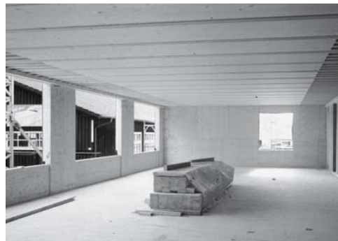
Fig. 274: Seminar room prior to fitting-out work The ceiling comprises Lignatur box elements left exposed which present a continuous soffit. This results in excellent flexibility for the positioning of partitions.
