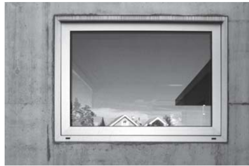
Fig. 110: Window flush with facade surface Fitting the window in this way calls for carefully controlled details in terms of sealing against driving rain and wind pressure (rebated joints).
