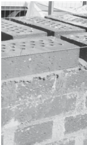
Fig. 84: Corner showing toothed intersection
