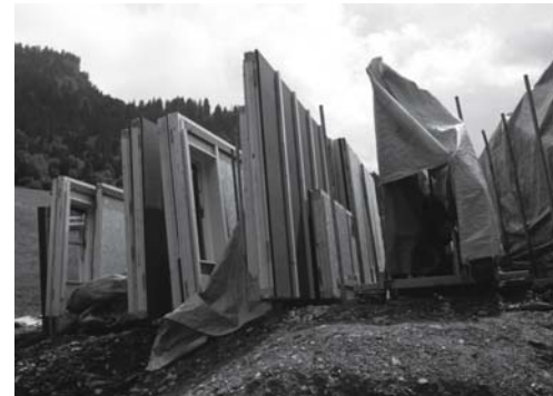
Fig. 297: Timber platform frame elements waiting to be erected The timber platform frame construction was erected in two days.
