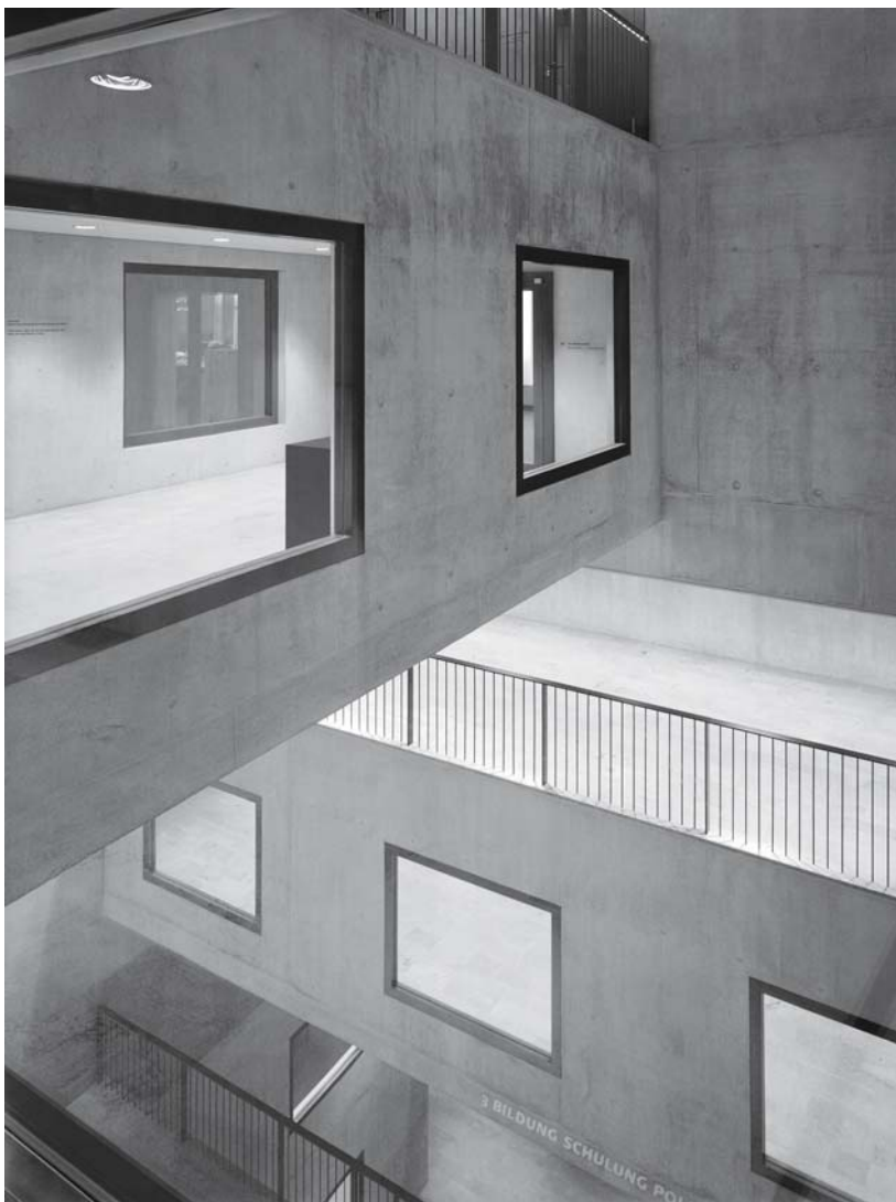
Fig. 192: Upper atrium, looking down towards entrance level The walls without intermediate supports act as storey-high deep beams.
