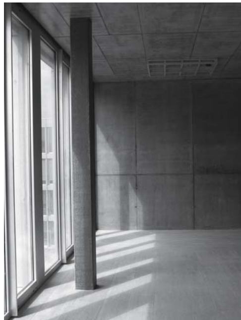
Fig. 216: Column and wall Access zone in secondary school, fair-face concrete wall with formwork type 2 and precast concrete column
