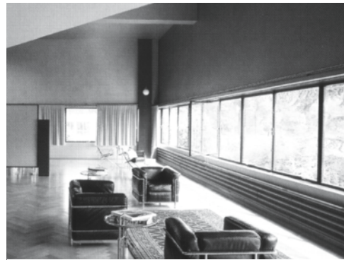
Fig. 16: Heating pipes grouped to form a surface Alexander Ferenczy, Hermann Henselmann: Kenwin Villa, Vevey (CH), 1929
