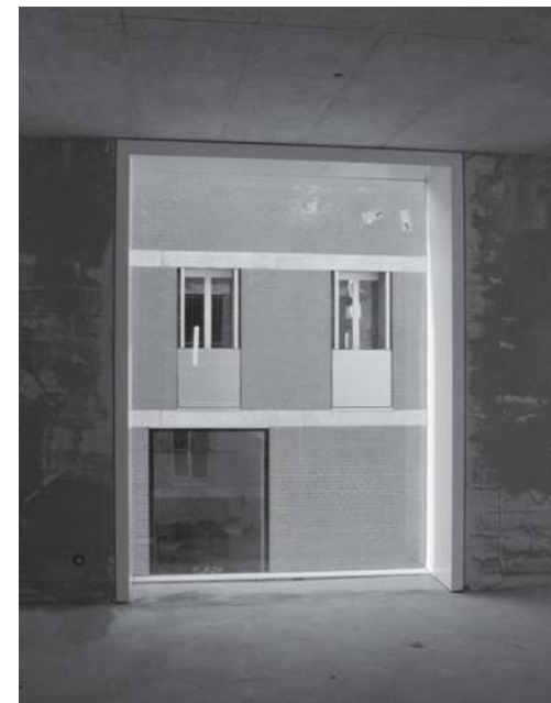
Fig. 58: View of “frameless” window from inside The reveals enable the thickness of the masonry to be appreciated.
