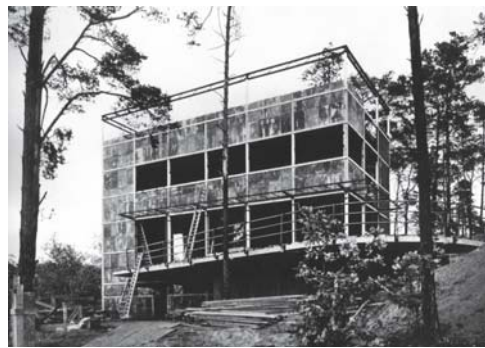
Fig. 10: Steel frame during construction Wassili and Hans Luckhardt: house on Rupenhorn, Berlin (D), 1928
