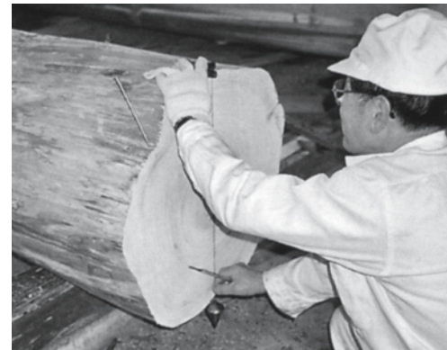
Fig. 54: The master carpenter at work Marking the end of a trunk with a plumb line
