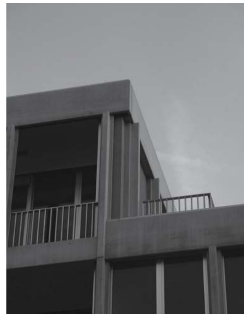
Fig. 220: Corner of building and edge of roof Steel safety barrier to escape balcony, glazing and rendered brick wall
