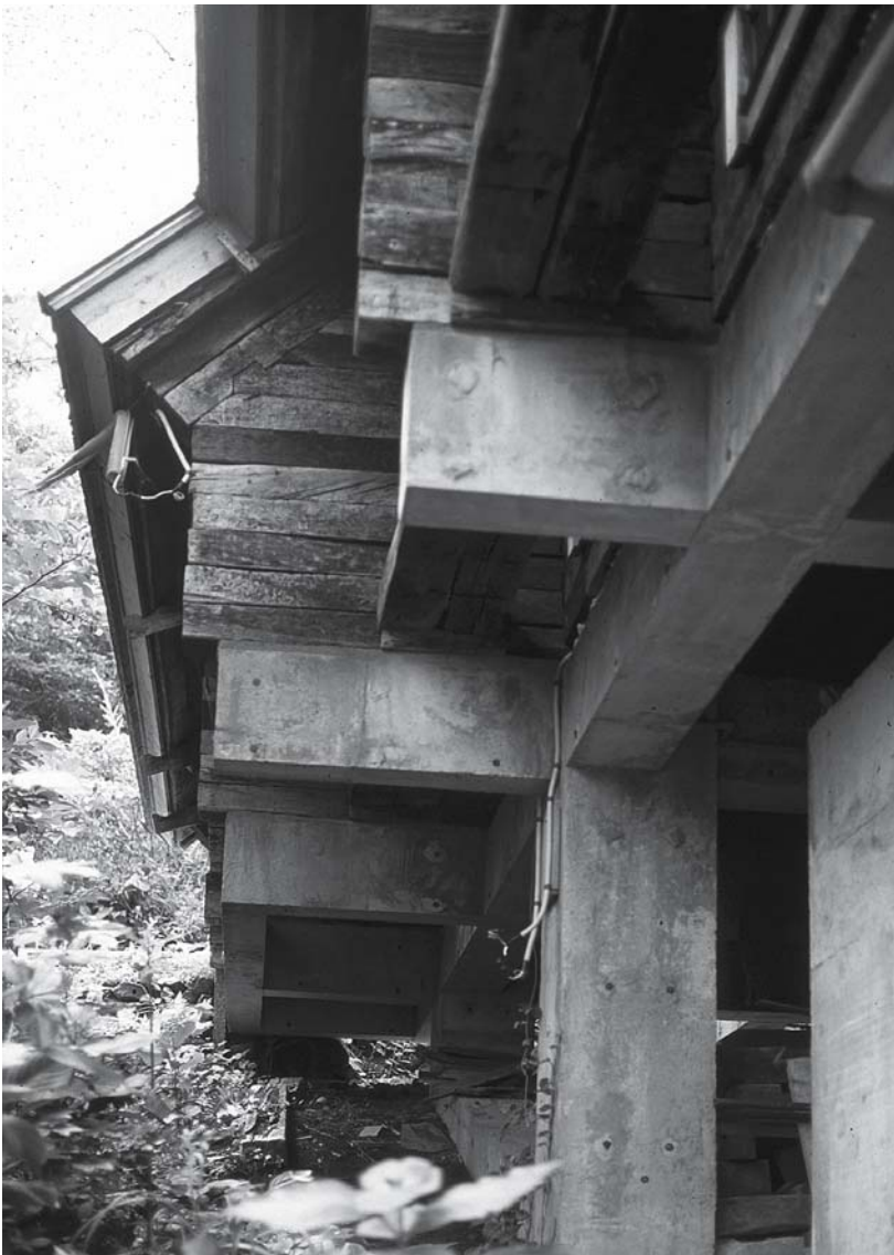
Fig. 72: The concrete substructure beneath the log construction superstructure Shin Takasuga: "Railway Sleeper House", Miyakejima (J), 1980
