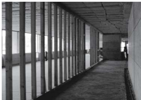
Fig. 273: Transition between concrete core and timber box The timber and concrete parts are structurally independent systems. The timber studding is covered on the corridor side with a cement fibreboard (Duripane) for fire protection purposes.
